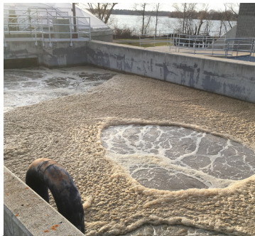
Activated Sludge Basin
