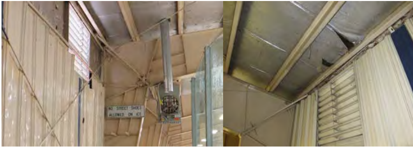
Picture Window 7 (l to r): Intake louver & gas fired heater, vapor barrier penetration, mold & rust
