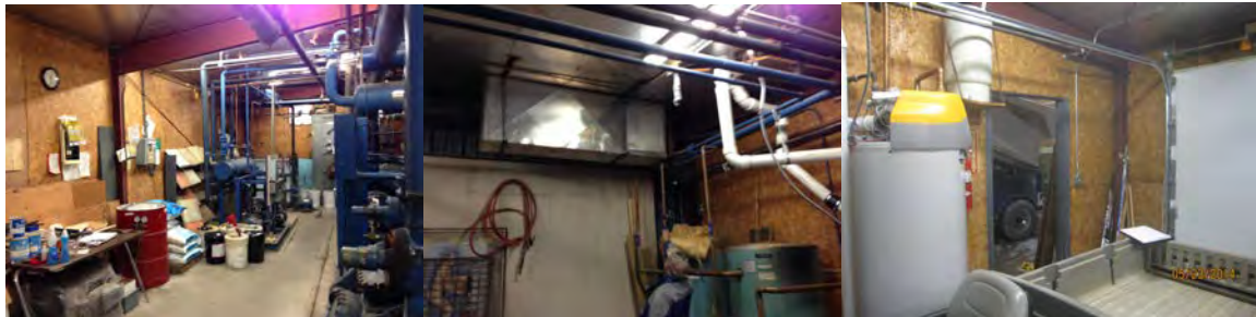
Picture Window 4 (left to right): interior of refrigeration room
