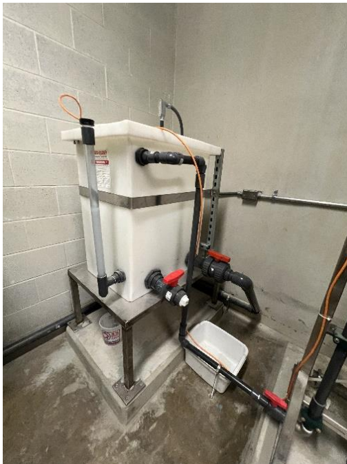
Figure 11: Thursday, August 28 th , raised polymer feed tank.
