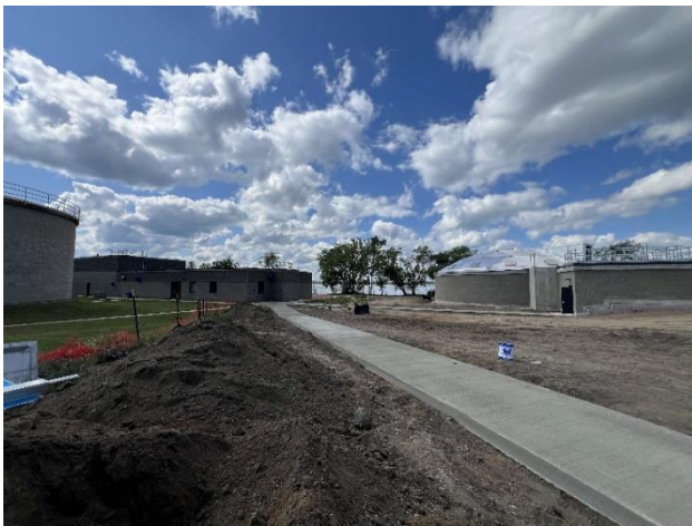
Figure 11: Thursday, July 17 th , poured sidewalks on the west side of the construction area.
