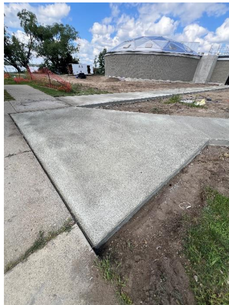
Figure 12: Thursday, July 17 th poured sidewalks on the west side of new secondary gallery.
